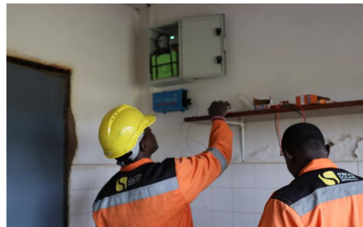
Figure 6 : Installation of the Wata Kit at the Mataketa health centre
