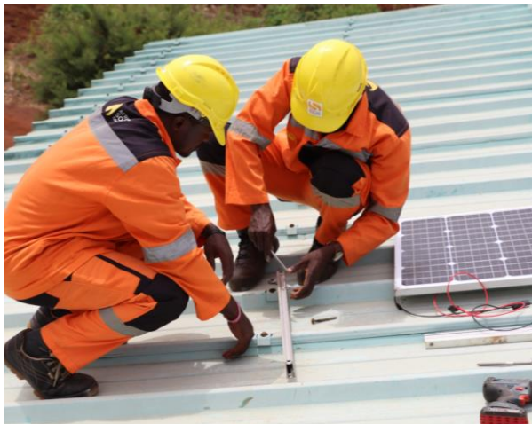
Figure 3 : Installation of the solar panel supplying the Wata Kit with electricity
