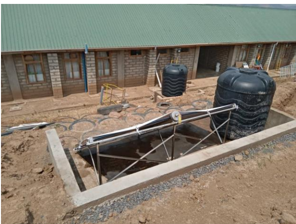
SoWaDis system safewater tank and in the background the rainwater tank
