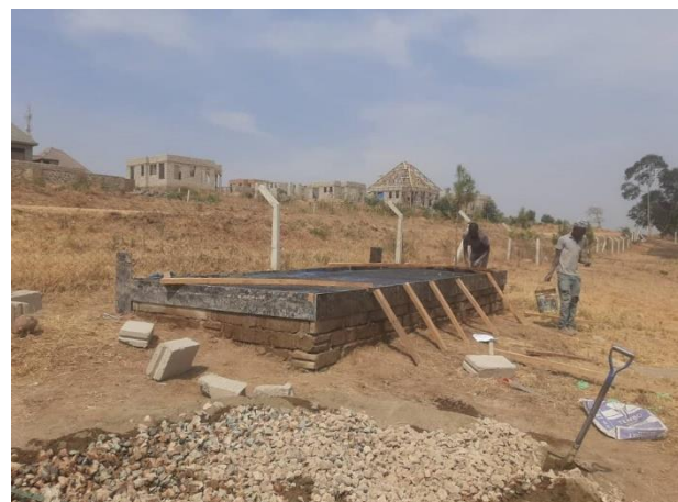
Large platform for the two water supply tanks
