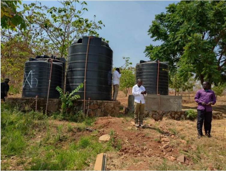
Starting point for the school's water supply: centralised tanks supplied with water from the borehole. The two SoWaDis systems obtain the raw water from here.
