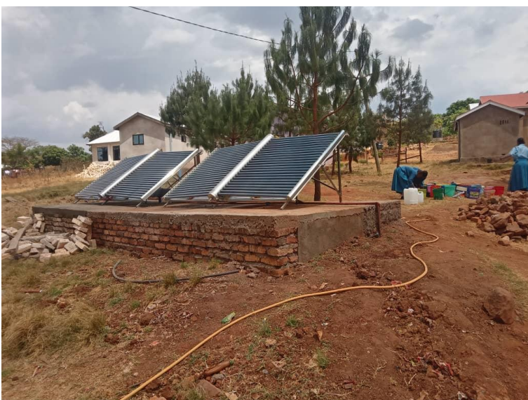
The platform extended with two SoWaDis systems.
