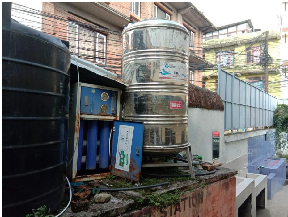
Water purification RO system, water tank, and drinking water station
